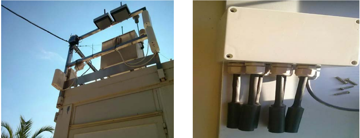
Figure 1. (a) Palau Reial reference Station, (b) CAPTOR node with 5 ozone sensors, and 1 Temperature/Humidity sensor
