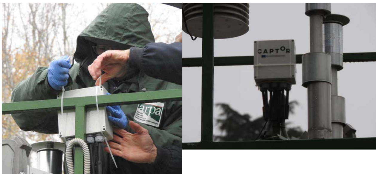
Figure 5: Captor nodes installation in Official Monitoring station in Italy
